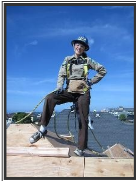
Brittany Higgins, CCC, exemplifies the triumphant spirit of community atop the new roof of the Annie B. Ryan.
